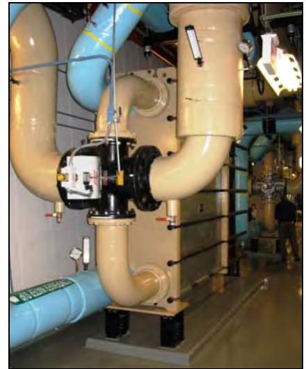
Times Square High-Rise Three Parallel Chilled Water Economizers MODU-FLEX™ Model MFK101 - 10" ports With Diverter Valves & Controls Design Pressure: 150 PSIG Heat Transfer Area: ~ 10,000 ft 2
