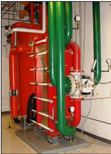
Major US City Business Center Cooling Tower Isolation MODU-FLEX™ Model MFK063 - 6" ports With Diverter Valves & Controls Design Pressure: 300 PSIG Heat Transfer Area: ~ 1,800 ft 2
